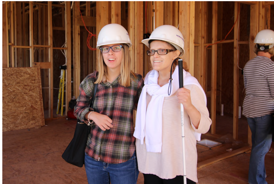
From left: Lyndsey Eaton and Lauren Heimerdinger, future residents, check out the First Place-Phoenix construction site in 2016.
